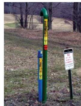
Pipeline markers are required by federal law and it is a crime to tamper with them.
